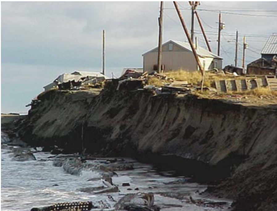
Figure 4: Bluff Erosion and Permafrost Melting in Shishmaref c. 2002 (Source: Kawerak)
