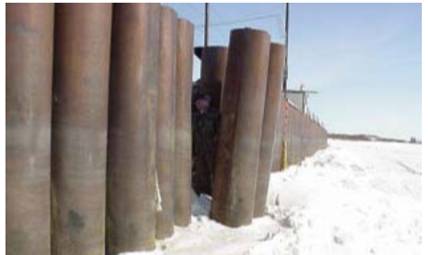
Figure 9: Pile wall of current concern at Bethel (Source: Army Corps)
