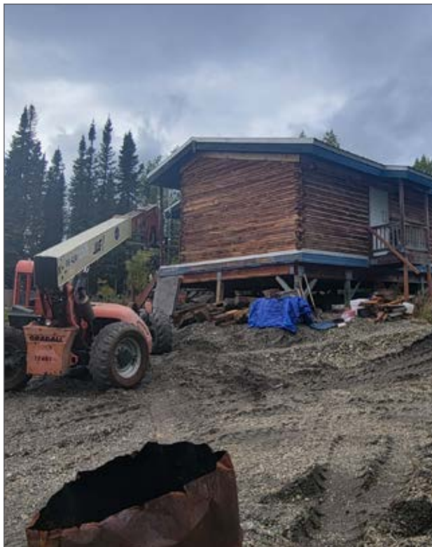
Foundation remediation in Alatna due to erosion. Photo courtesy of Jonathan Henzie
