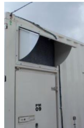
Hood to protect air intake.
