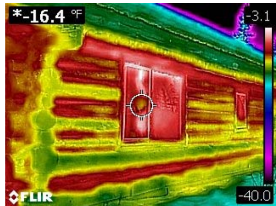
FLIR thermal imaging of the Venetie IGAP/ICWA Building's broken window. The colors on the higher end of the color gradient scale indicate areas that have greater heat loss.
