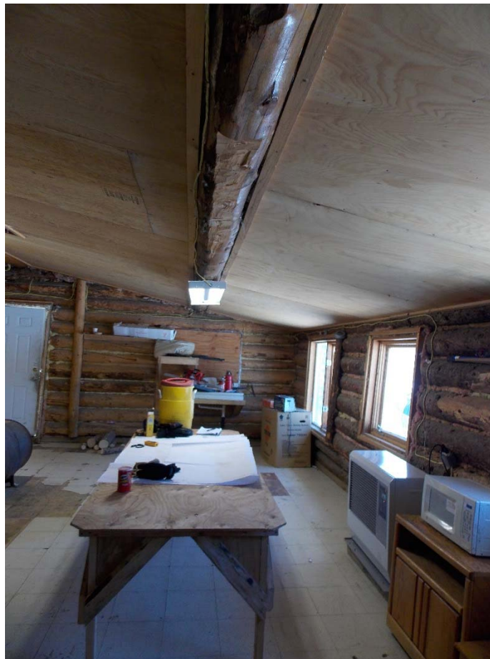
Building interior. The main entrance door on the left has gaps between the door and the header. Weather stripping should be applied to the door frame and spray foam added around the frame to reduce heat loss. The wall on the right is bowing toward the interior of the building.
