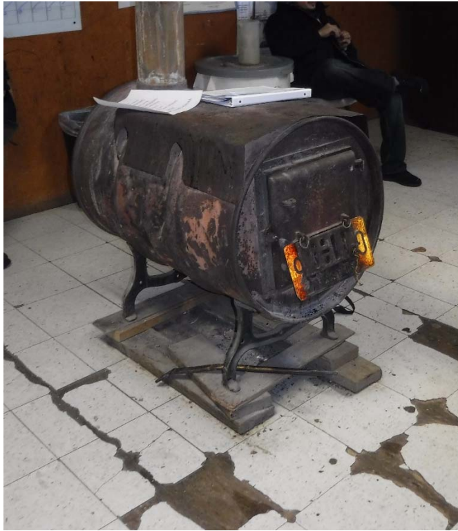
Council Office barrel-style wood stove.
