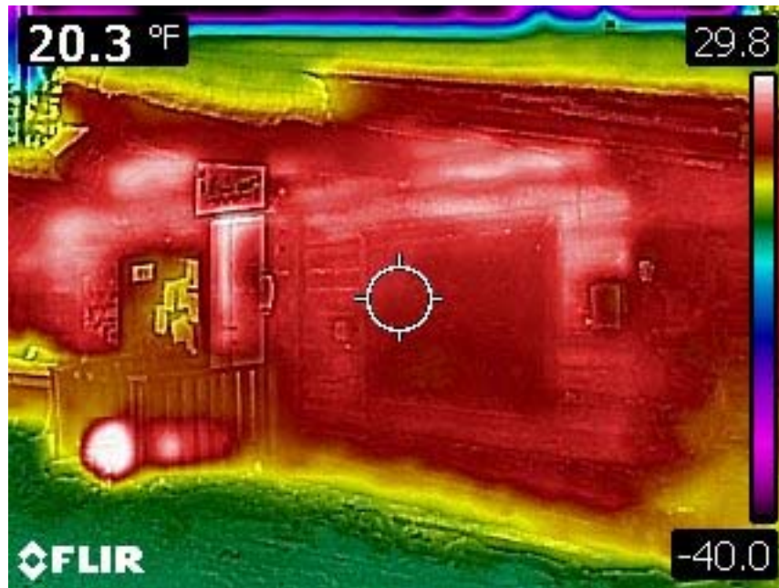
FLIR thermal imaging of the Council Office main entrance. The color gradient on the right depicts the temperature range of the photo (-40° F to 29.8° F). Colors in the higher end of the gradient indicate where heat is being lost.
