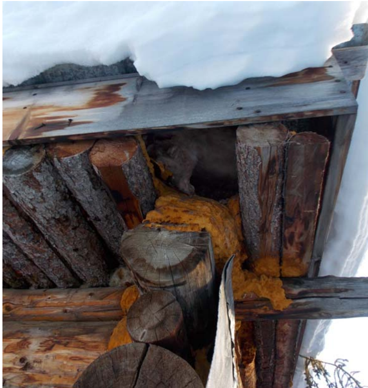
Building's current roof. Gaps at the eaves and corners of the roof expose the fiberglass batt to moisture. Moisture damages the batt, reducing its ability to insulate the building.
