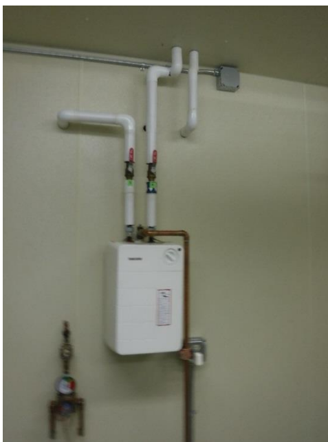
Figure 14: Hot Water Heater
