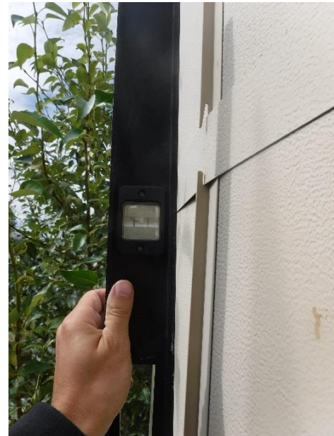
Figure 6: Level indicator showing the approximate tilting angle of the uphill side of the water storage tank.
