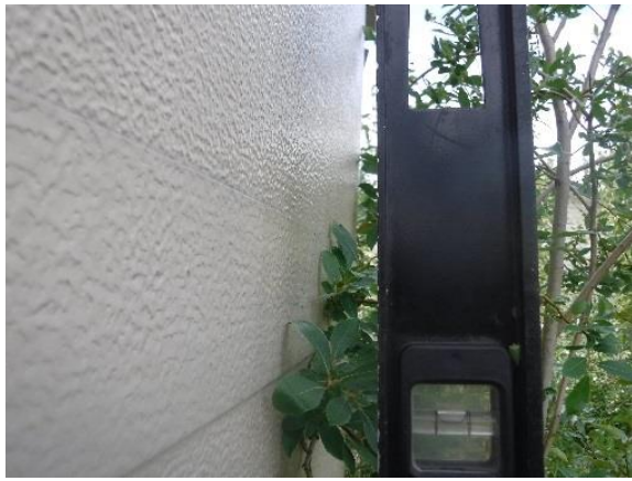
Figure 5: Level indicator showing the approximate tilting angle of the downhill side of the water storage tank.
