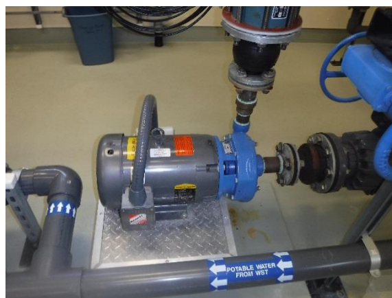
Figure 20: High Capacity Pump
