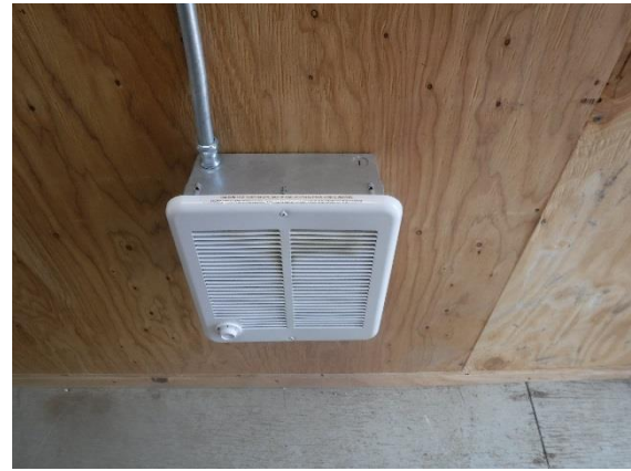
Figure 12: Old Water Treatment Plant Space Heater
