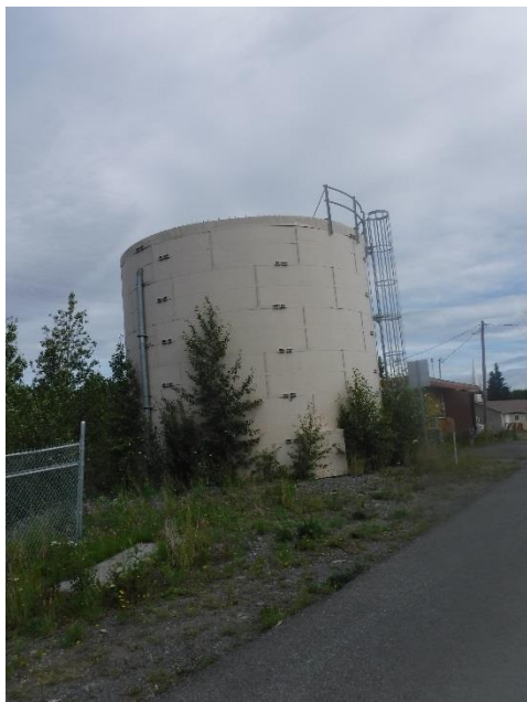
Figure 3: Water Storage Tank shown leaning to the left
