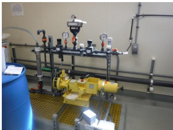
Figure 19: Chlorine Injection Pump
