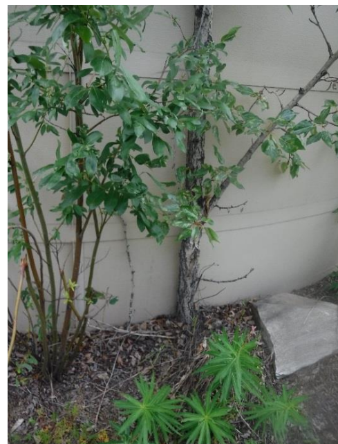
Figure 4: Trees growing in the water storage tank foundation, creating instability in the foundation soil
