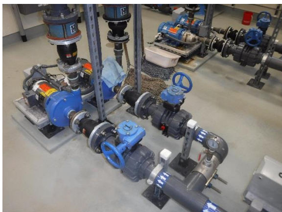
Figure 21: Distribution Loop Circulation Pumps
