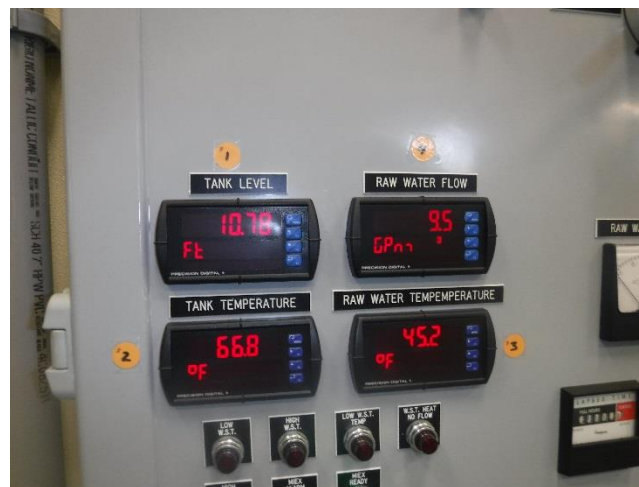
Figure 7: Raw Water Intake GPM and Water Storage Tank Water Level during the Site Visit
