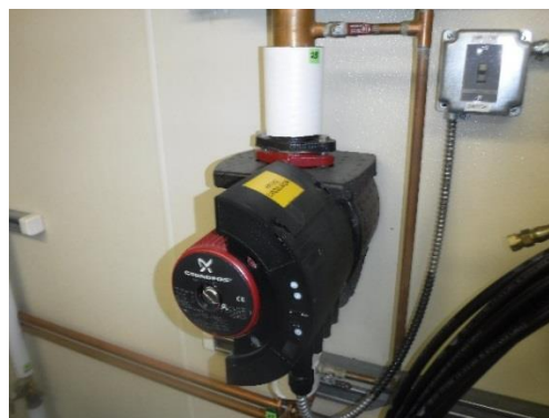
Figure 13: Heating Circulation Pump
