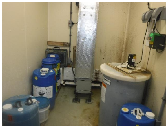
Figure 16: Chemical Room Exhaust Fan
