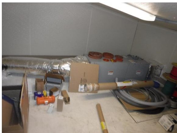
Figure 15: Boiler Room Exhaust Fan
