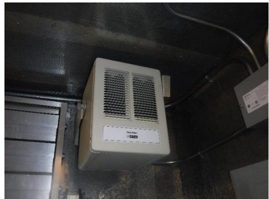
Figure 10: Generator Unit Space Heater
