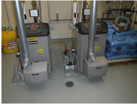
Figure 8: Water Treatment Plant Boilers
