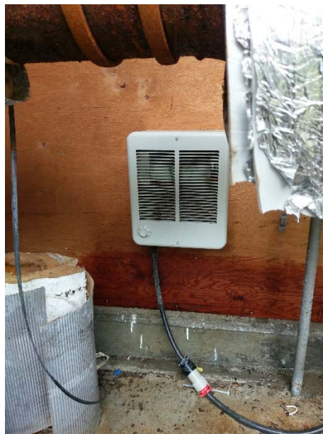
Figure 6: Well House 2 heater.
