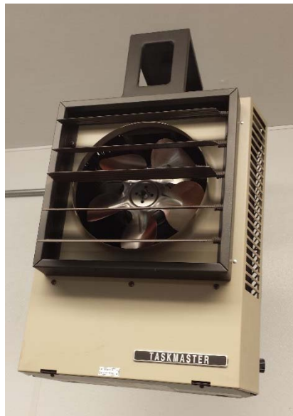
Figure 4: Pump Room unit heater in the Water Treatment Plant.
