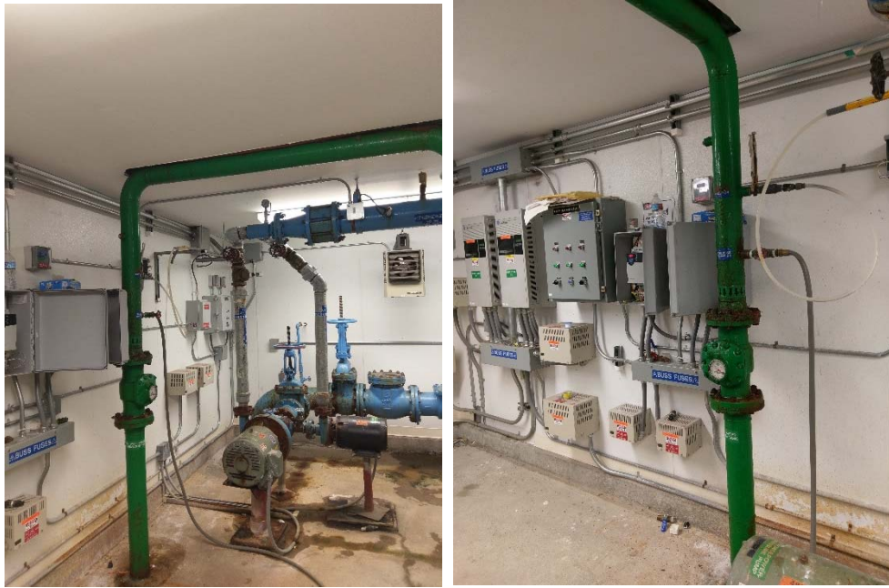
Figure 14: Water Treatment Plant Pump Room interior.
