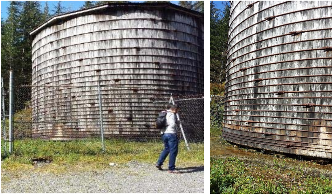
Figure 2: Wood Stave Water Storage Tank near the Water Treatment Plant. The image on the right shows the rapid rate of water loss through the bottom and sides of the tank.
