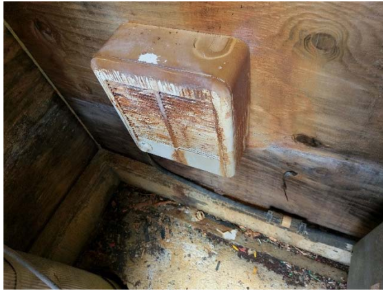
Figure 5: Well House 1 heater.
