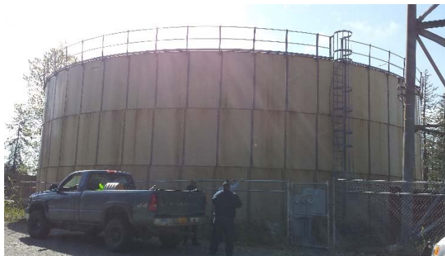
Figure 3: 1 Mil Water Storage Tank.
