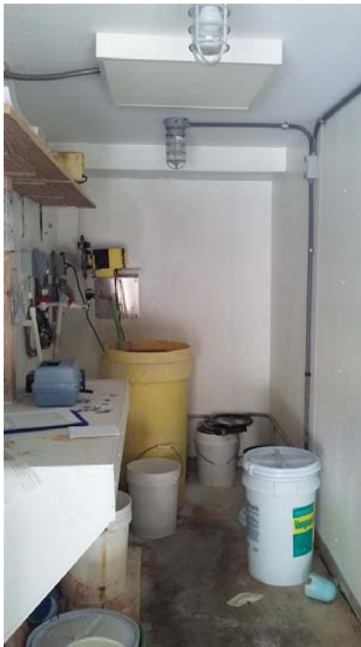
Figure 15: Chemical Injection Room interior. The ceramic unit heater is the square object attached to the ceiling.
