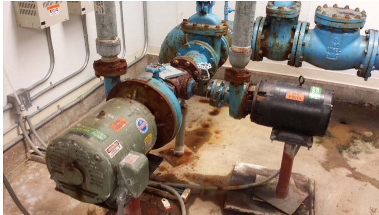
Figure 7: 15 HP (left) and 10 HP (right) pressure pumps in the Pump Room in the Water Treatment Plant. The 10 HP pump is rarely used. The blue turbine at the top of the photo sends water to the fish processing plant.
