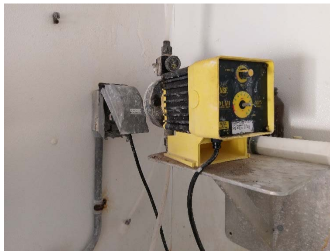
Figure 8: Chlorine pump in the Chemical Injection Room at the Water Treatment Plant.
