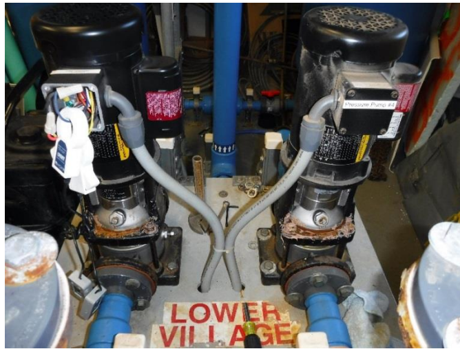
Figure 9: Lower Village Pressure Pumps
