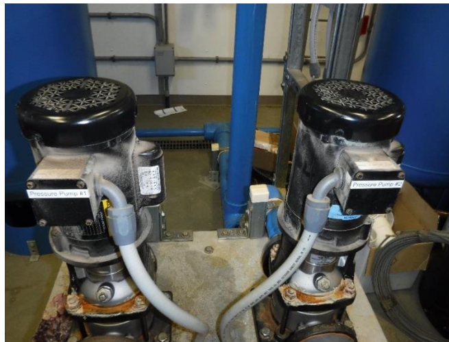
Figure 8: Indian Creek Pressure Pumps
