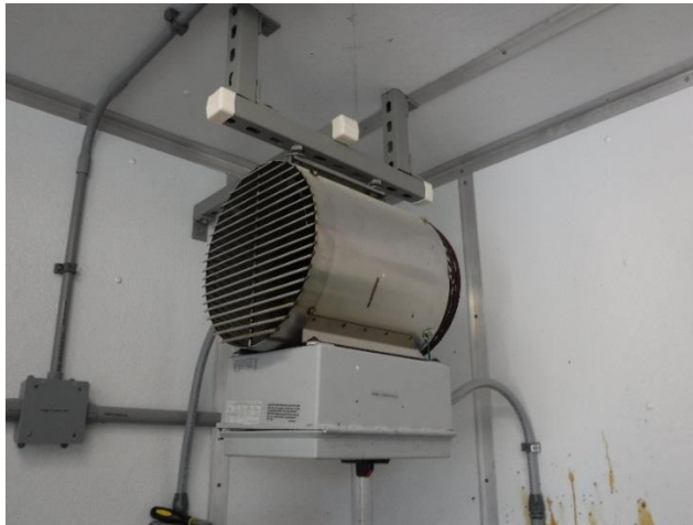
Figure 5: Chemical Room Electric Heater
