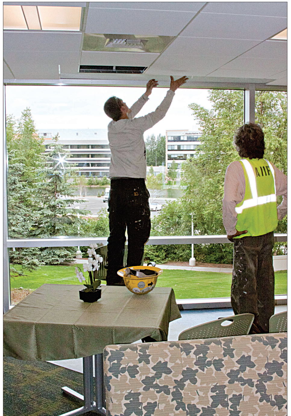
PHOTO BY TODD HENRY / ANTHC Construction teams put the finishing touches on the new gathering area in the Quyana House at the Alaska Native Medical Center.
