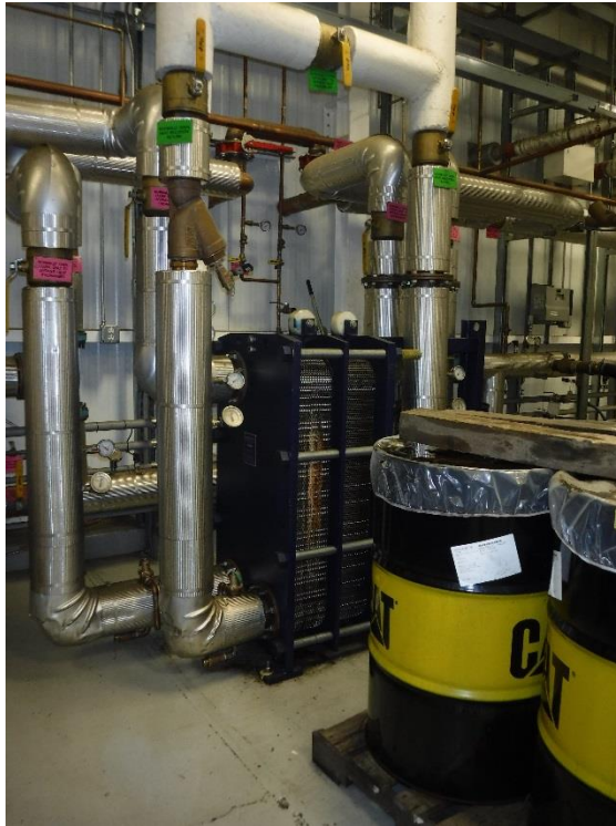
Figure 6: Heat Recovery Heat Exchanger in the Power Plant
