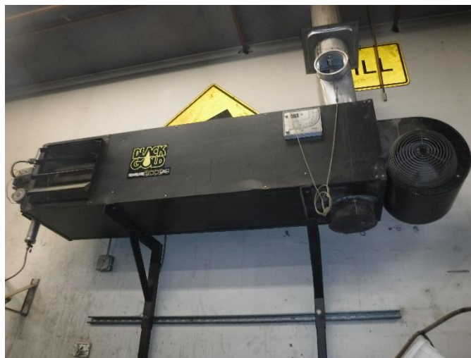
Figure 7: Waste Oil Space Heater in the Middle Garage
