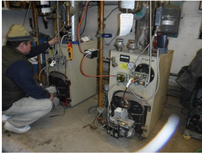
Figure 4: Boiler 1 (Left Side)
