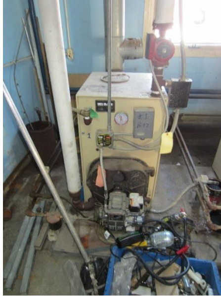
Figure 6: Middle Pump House Boiler 1
