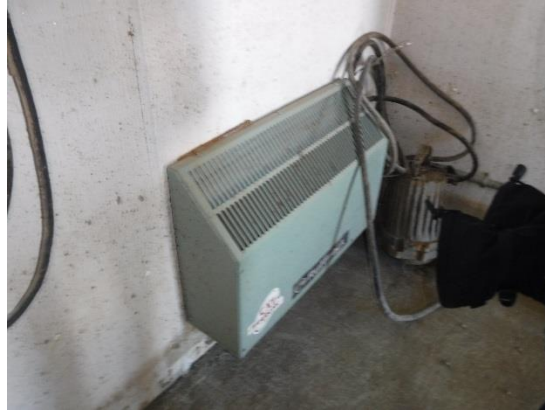
Figure 11: Lift Station 2 Electric Heater
