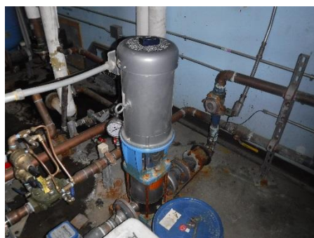
Figure 13: Middle Pump House Transfer Pump
