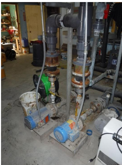
Figure 12: Middle Pump House Circulation Pumps
