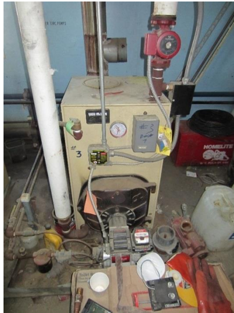
Figure 8: Middle Pump House Boiler 3
