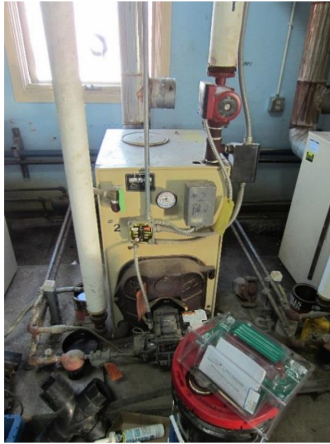
Figure 7: Middle Pump House Boiler 2
