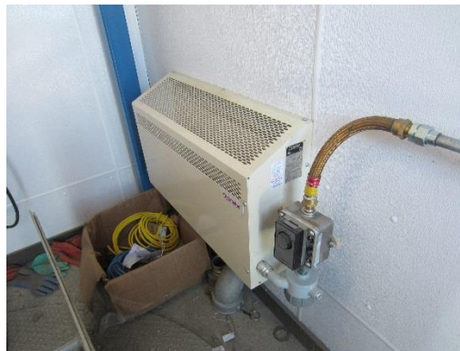
Figure 10: Lift Station 1 Electric Heater
