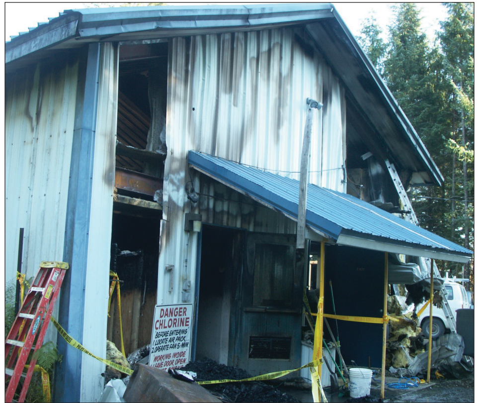
Klawock's fire-damaged water treatment plant.
