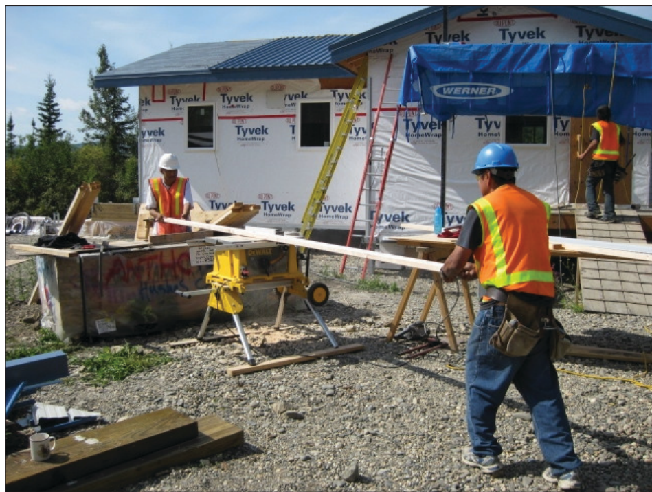
A local work crew helps construct a health clinic in Hughes, Alaska. JC CRAWFORD PHOTO
