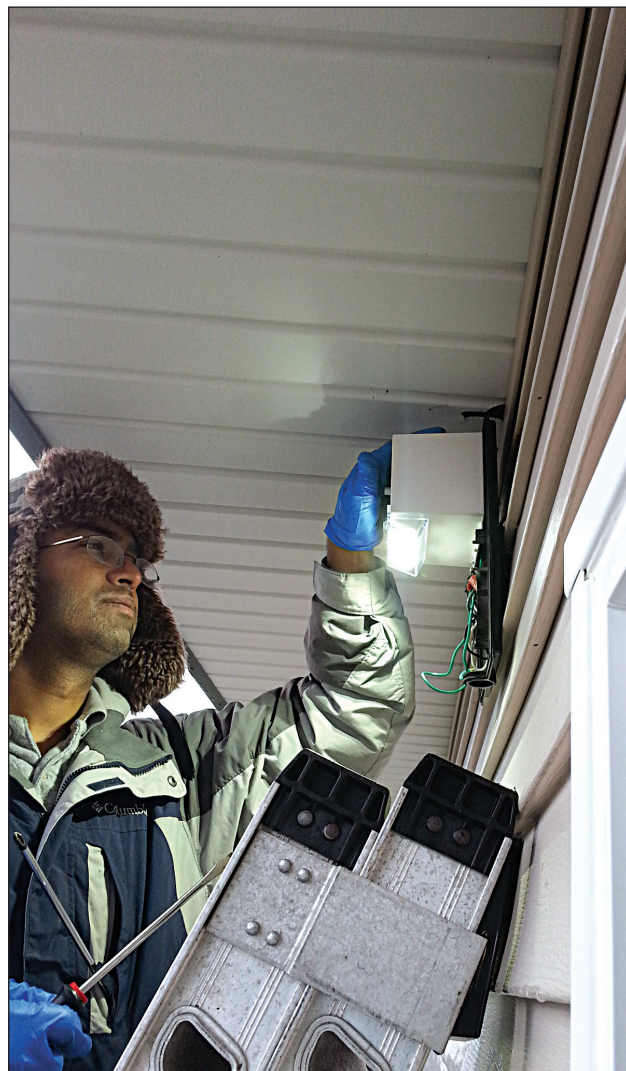
ANTHC Mechanical Engineer Praveen K.C. evaluates new LED lighting installations in Nulato.
