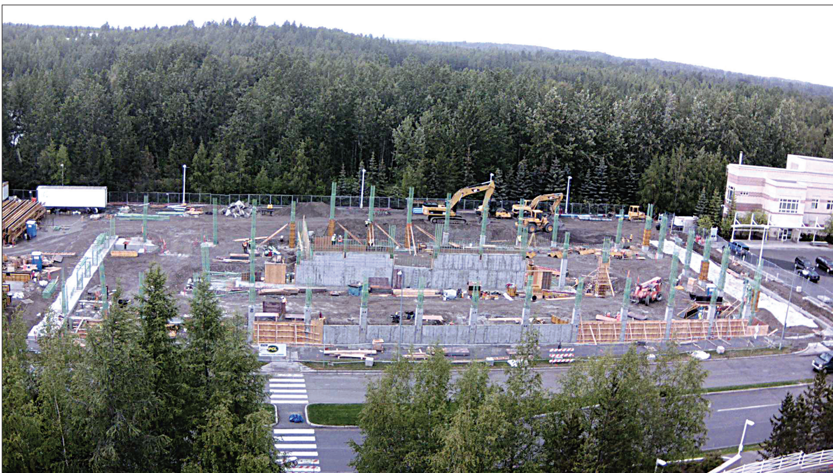
Construction is well underway at the site of the new ANMC parking garage.
