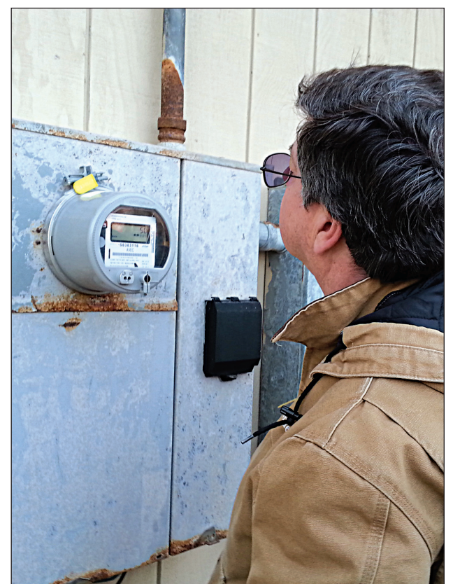
ANTHC Consulting Engineer Carl Remley analyzes electric meter data in Marshall.
