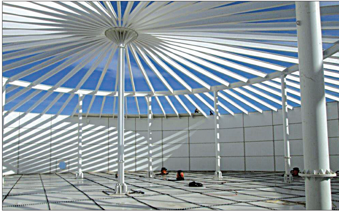
A new water storage tank and a water treatment plant are being built in Golovin.
