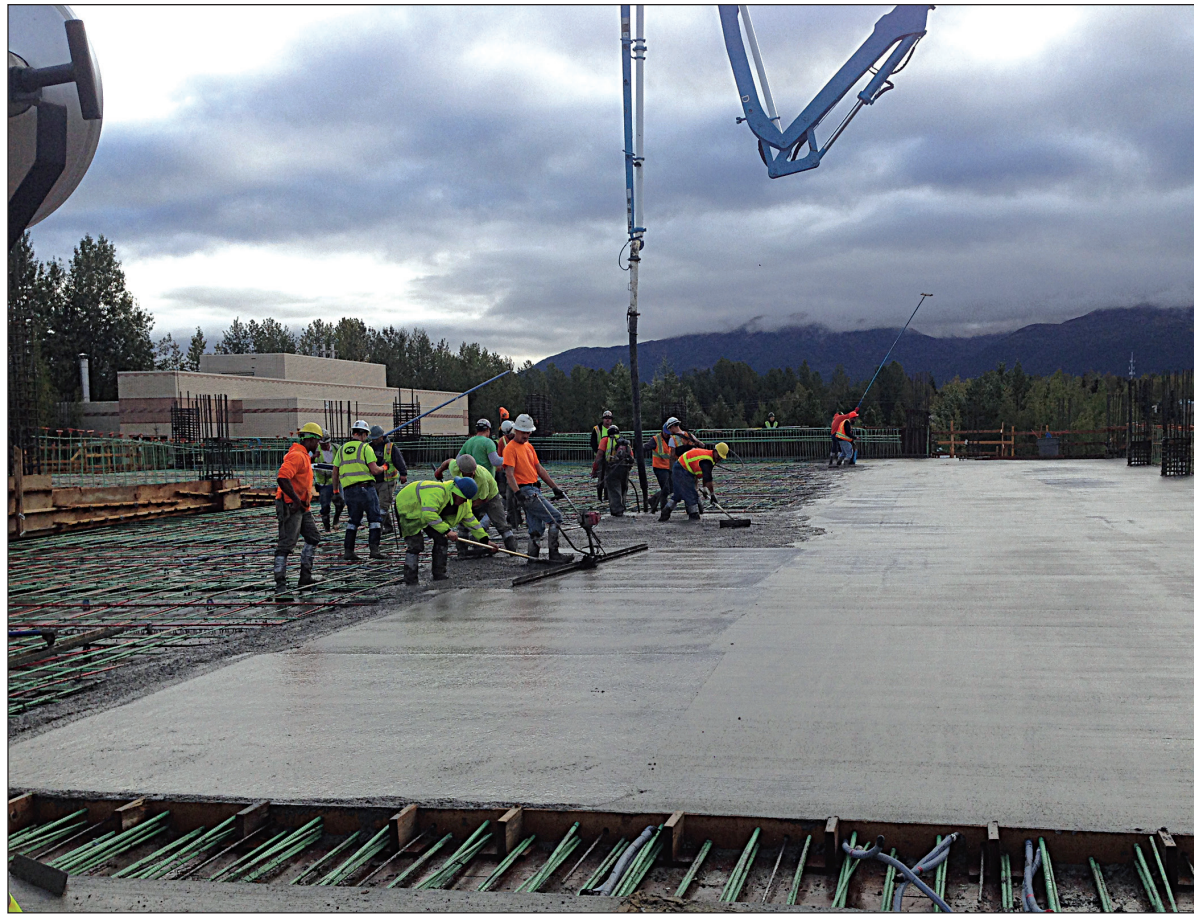
Construction workers recently put the finishing touches on the third floor of the new Alaska Native Medical Center hospital's parking garage.
