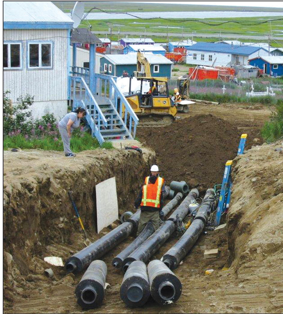
Work crews install water lines in Scammon Bay. The work is part of a large project which includes a new water treatment facility for the community.
