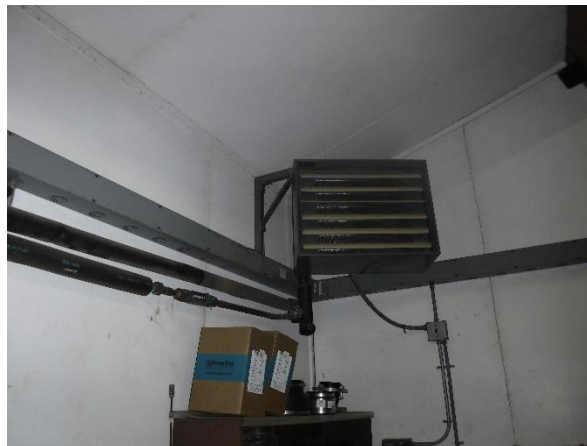
Figure 12: Unit heater located in the upper corner of the water treatment plant
