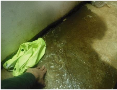
Figure 4: Ice is shown near the bottom of the exterior walls where the insulation has been damaged.
