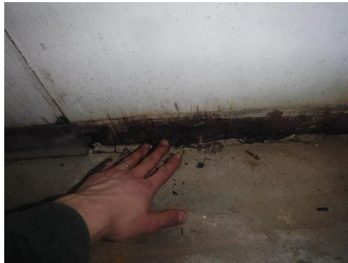
Figure 5: The damaged insulation in the exterior wall can be seen near the ground level.
