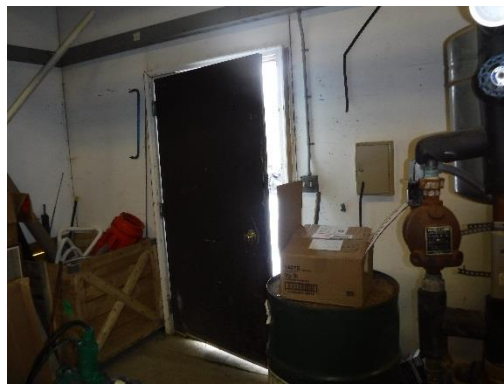
Figure 8: The front entrance door after it had been closed without a padlock. It cannot remain closed without a padlock.
