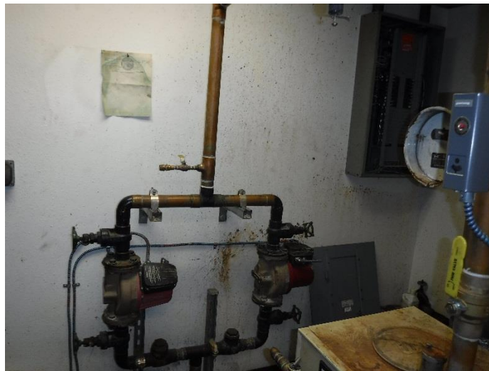
Figure 11: Heat Circulation Pumps in the Circle Washeteria
