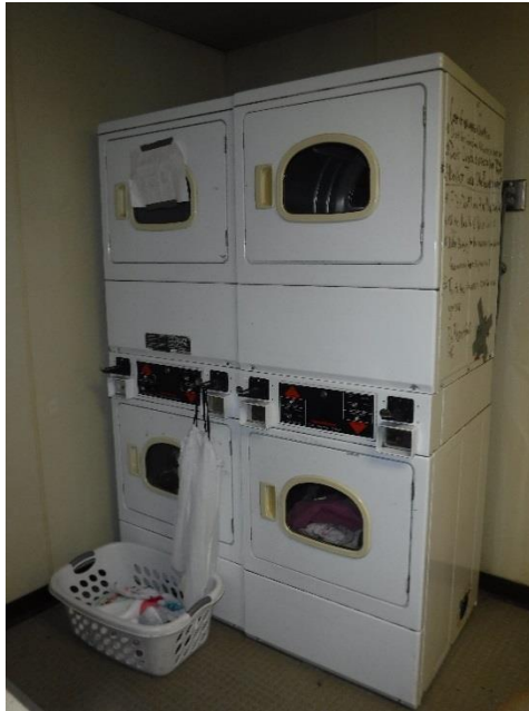
Figure 12: Propane Clothes Dryers in the Circle Washeteria
