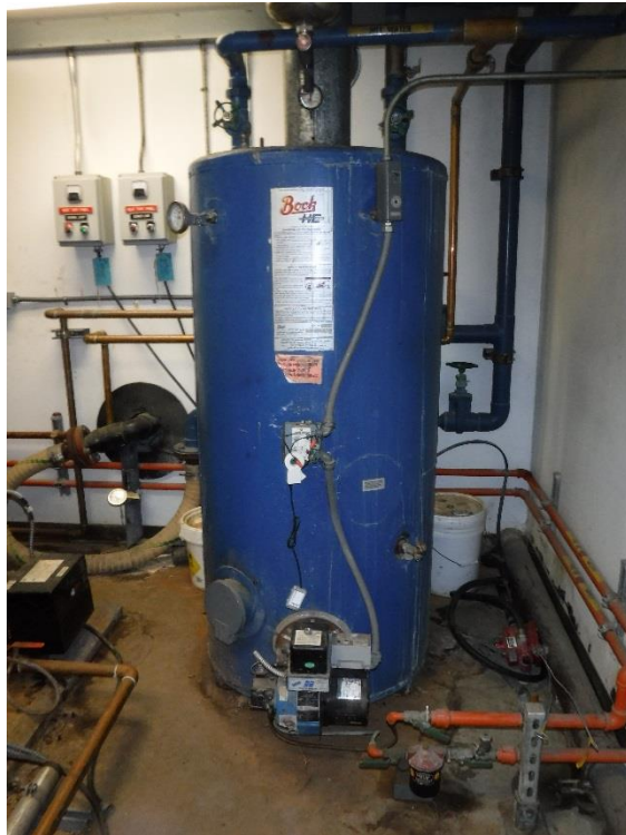
Figure 2: Hot Water Heater in the Circle Washeteria
