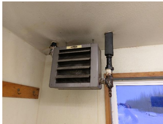
Figure 7: Functional Unit Heater with leaks in the Circle Washeteria
