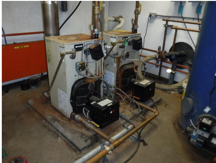
Figure 1: Fuel Oil Boilers in the Circle Washeteria
