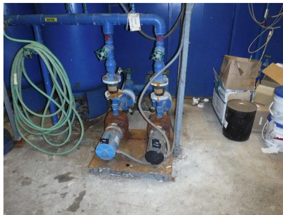
Figure 9: Pressure Pumps in the Circle Washeteria
