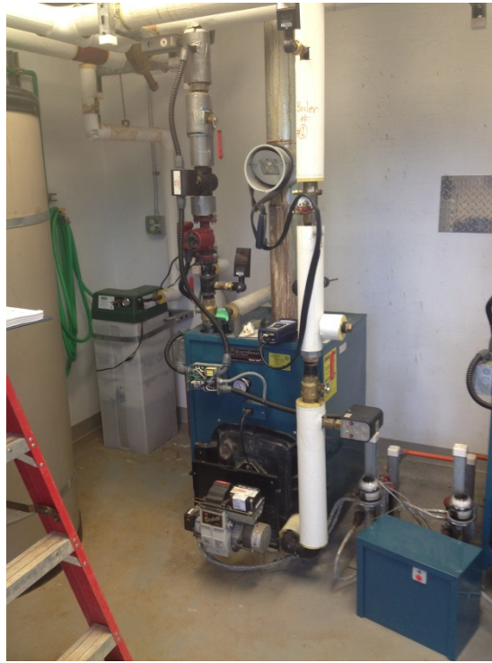
Sand Point Mechanical Room
