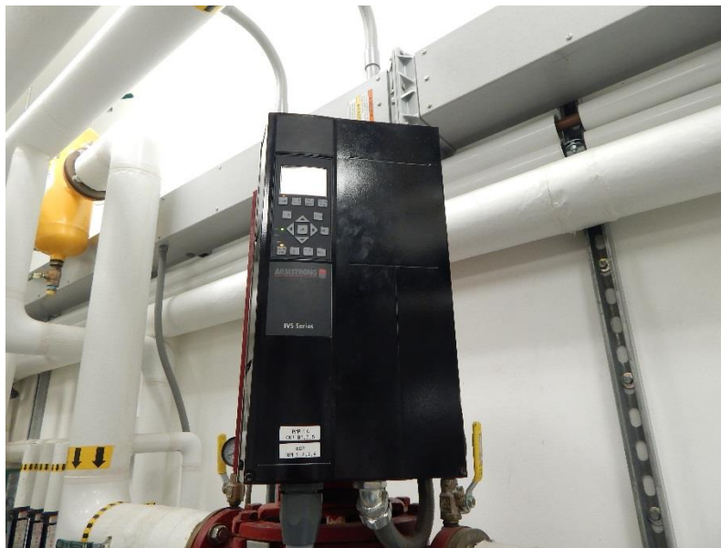
Figure 4.1: Glycol Circulation Pump
