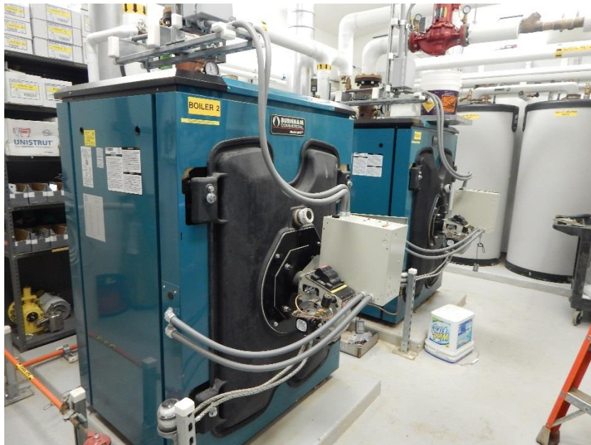
Figure 3.1: Burnham Boilers in the Mechanical Room
