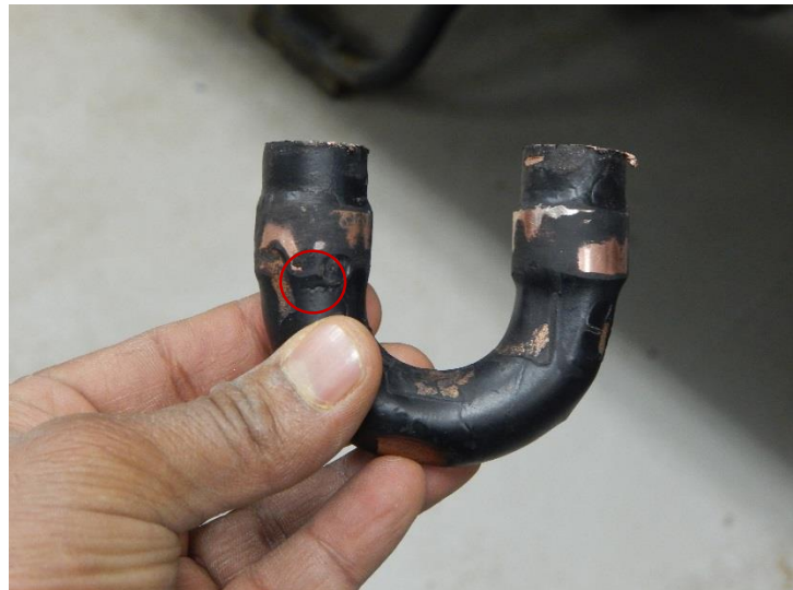
Figure 4.3: Hole in the Heat Exchanger Turn
