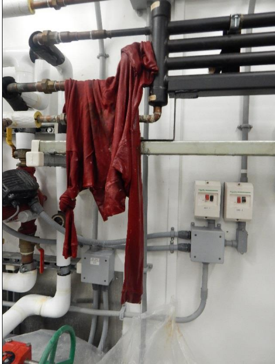
Figure 4.2: Leaks from the Water Storage Tank Heat Exchanger
