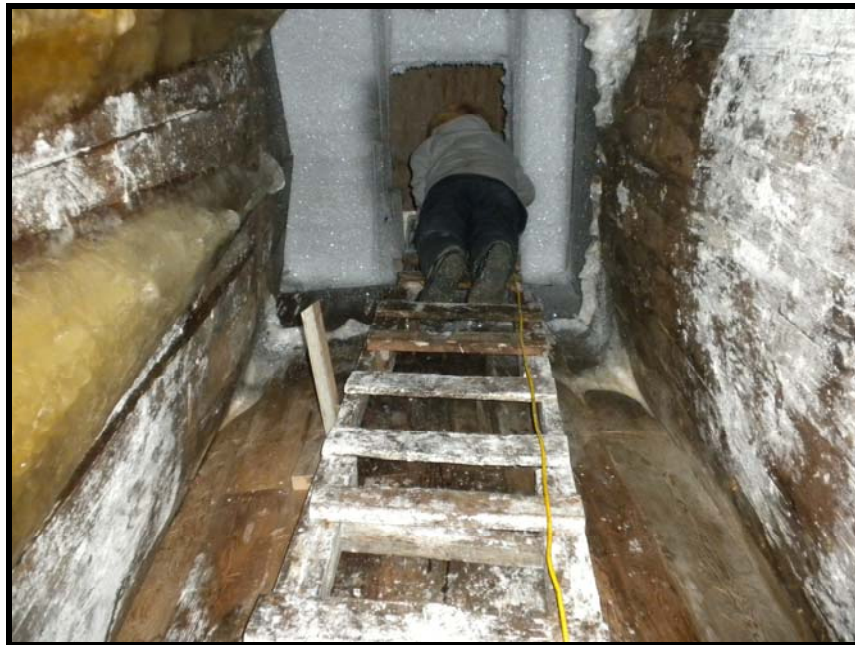
Price Leavitt inspects the condition of a cellar shaft and walls. (M. Brubaker, 2010)
