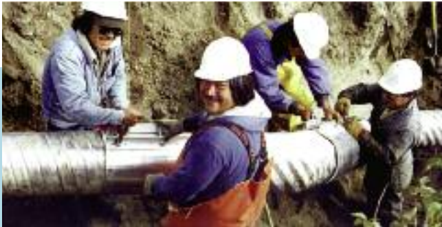
Division of Environmental Health and Engineering works on design and construction of sanitation facilities in more than 70 communities. In 2002, 6,000 homes were still without running water and sewer services.
